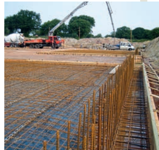
The 23cm deep concrete base for the underground slurry store was poured in square slabs with reinforcing bars protruding up to tie in the mass-poured concrete walls.
