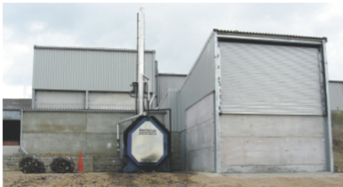
The Glenfarrow boiler, with Froeling boiler woodchip feeder shed (right) and tray drier to the rear at Balring.
