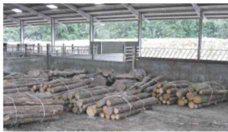
Bundled logs in the empty cattle shed waiting to be fed into the boiler.
