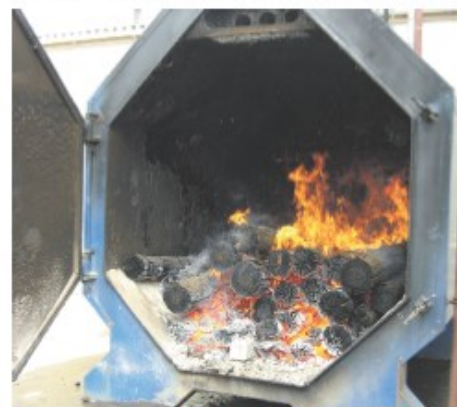
The original boiler is fed with bundles of logs produced at Baling.
